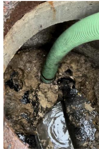
NWB Road sanitary sewer line blockage due to grease accumulation.
