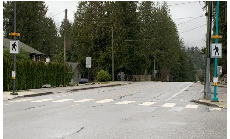
Bike BC project on Reef Road and RRFB Installation at NWBR/Emerson Intersection
