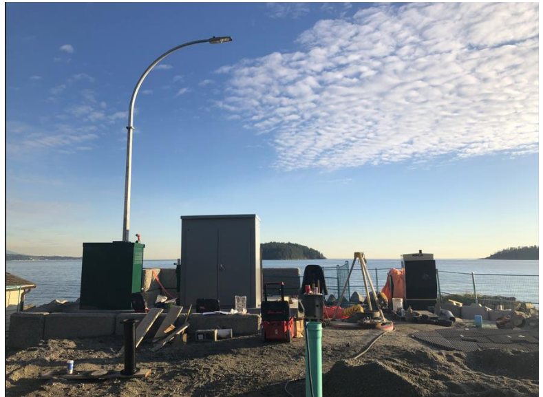
Wakefield Lift Station
