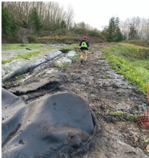
Stored septage solids, before removal.
