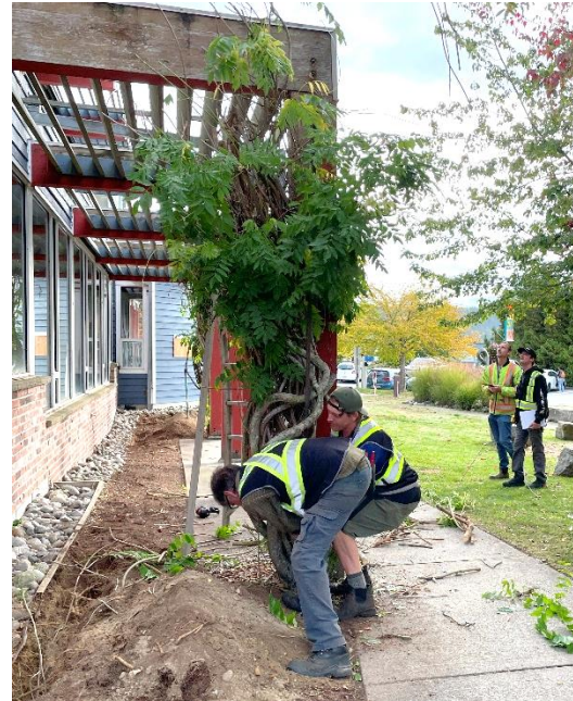
After: Much of the vegetation has been removed for building renovations. Staff did their best to preserve the wisteria.
