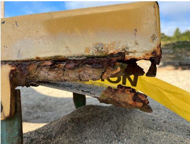
Before: rust damage to slide in Kinnikinnick Park
