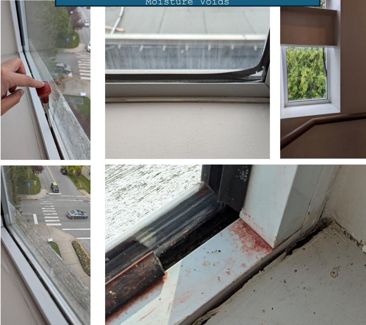
Deficiency Photos of Air Leakage and Moisture Voids
